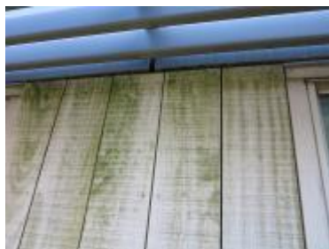
Figure 8: Moss and fungal growth on paint layer of wet timber.
