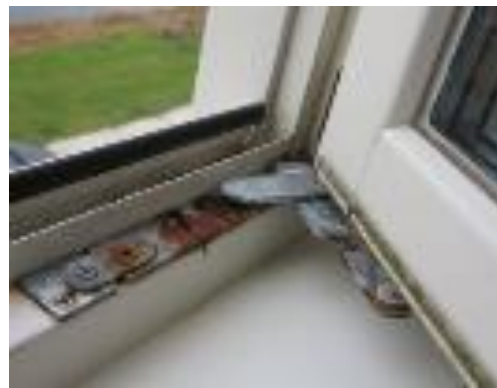
Figure: 4 Window with high and long term condensation causing corrosion on the metal parts.
