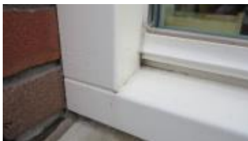
Figure 5: Joinery with small humps near the corner.
