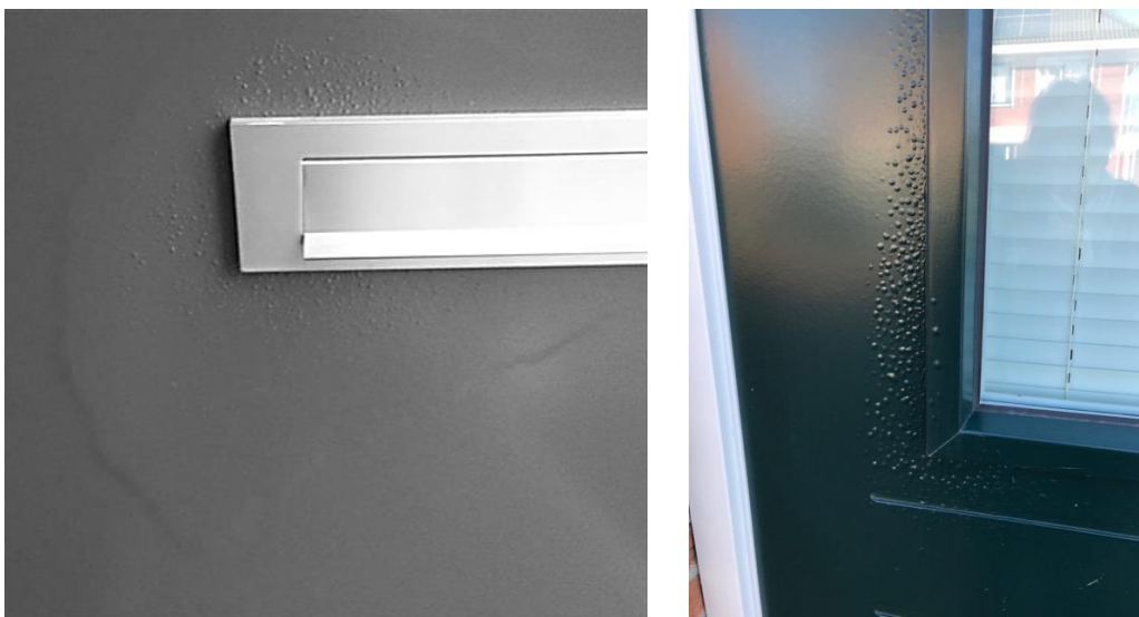
Figure 6: Left: swelling in a traditional exterior HDF door, Swelling trough capillary water from letterbox, also resulting in blistering in the paint. Right, detail of a glass bead on an A-MDF door, due to a failing seam there is water uptake in the panel. It does not show swelling, but blisters indicate paint film adhesion failure, after drying the paint adhesion can recover.
