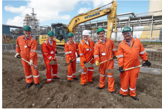
Figure 4: Breaking of soil for new acetylation plant for wood chips at Hull, UK
