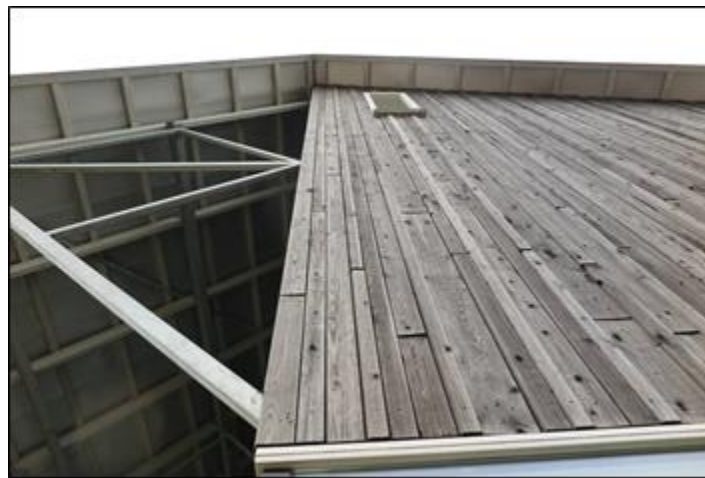
Figure 1: PPy 1.0 façade showing dimensional stability after four years of exposition on the south-west face of a detached house in Elden, NL (Picture: Innovita).
