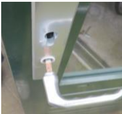
Figure 3: Sheet door which stood frequently open causing water accumulation in the lock resulting in corrosion on the metal parts.
