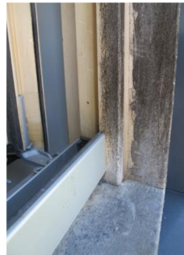
Figure 12: differences in discolorations and mould growth.
