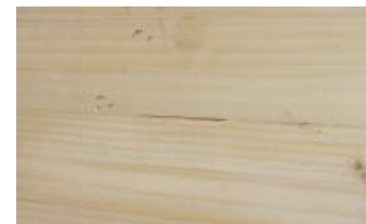
Figure 7: Beam in cycle track Assen with a removed shallow peel which was a result of a drying crack.
