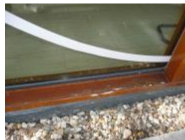
Figure 9: Window frame with high moisture content causing paint damage.
